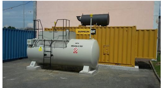
Figure 4. Diesel generator in container design with additional fuel tank
