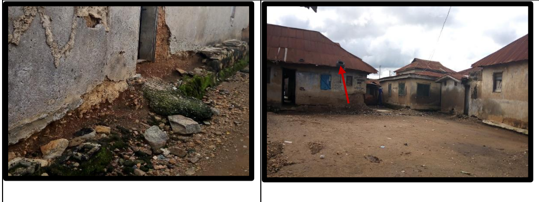
Figure 4: Typical buildings with eroded foundation and rustic roofs
