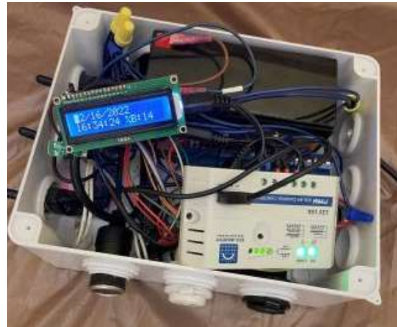
Fig. 7 Interior of junction box
