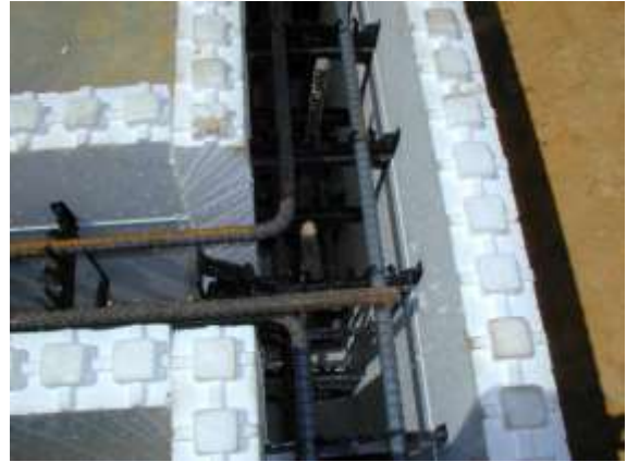
Fig. 46: Placing the T-wall forms together and tying intersecting blocks. Use metal or plastic wire ties supplied by Amvic
