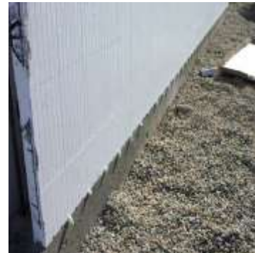
Fig. 36: Using foam adhesive to secure the first course of block to the foundation/slab
