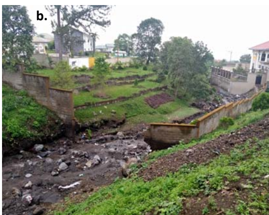
Fig.6. Physical impact of the 2020 flash floods on buildings represented on: a. pie chart and b. damaged wall at Federal Quarters (Mountain Hotel Area)
